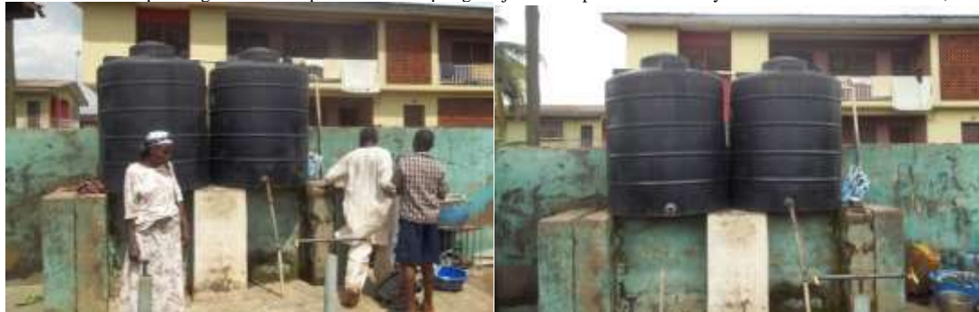
Plates-2. Upscaling Items at Onipasan Natural Spring Project at Onipasan Community Source: Author's Fieldwork, 2017
